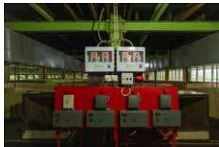
Digital hygrometer system installed at Gouravilla Tea Processing Center.
