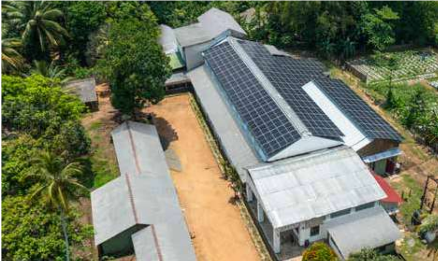
Factory rooftop solar installed at Frocester
