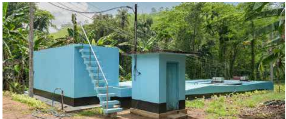
Wastewater treatment plant at Frocester Estate rubber processing unit
