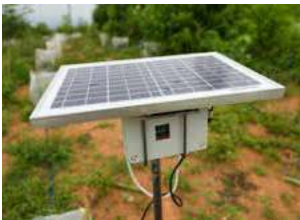
Smart weather station installed at Stockholm Estate.
