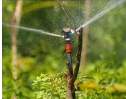
Sprinkler Irrigation System Implemented as a Water-Efficient Irrigation Practice
