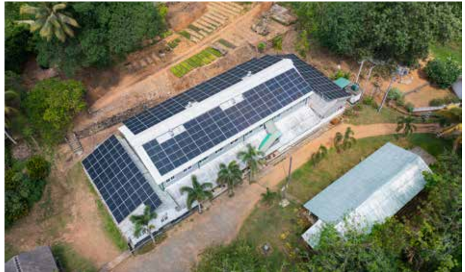
Factory rooftop solar installed at Kobowela
