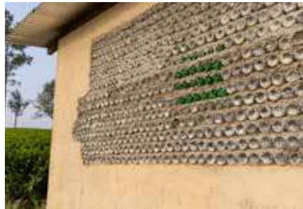
PET bottles are used as building material to promote recycling and reduce plastic waste, supporting sustainable and eco-friendly construction practices using the no of bottles 2620.
