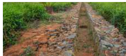
Drainage and sediment control system introduced at Millakande Estate enhancing environmental protection and soil conservation.
